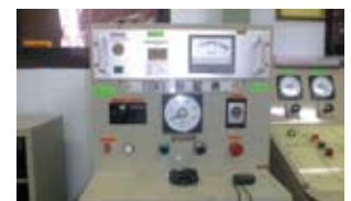
AC VOLTAGE WITHSTAND TEST EQUIP.
